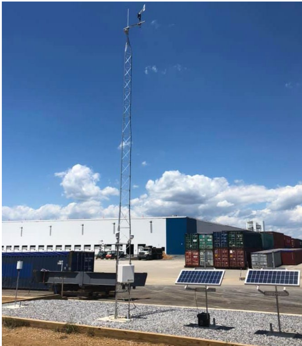
Figure 4: ROCKWOOL Meteorological Monitoring Location
